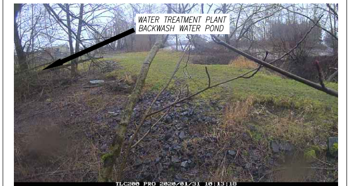
SCoured LEVEE BACKSLOPE BEFORE FLOOD - FEB 2020
