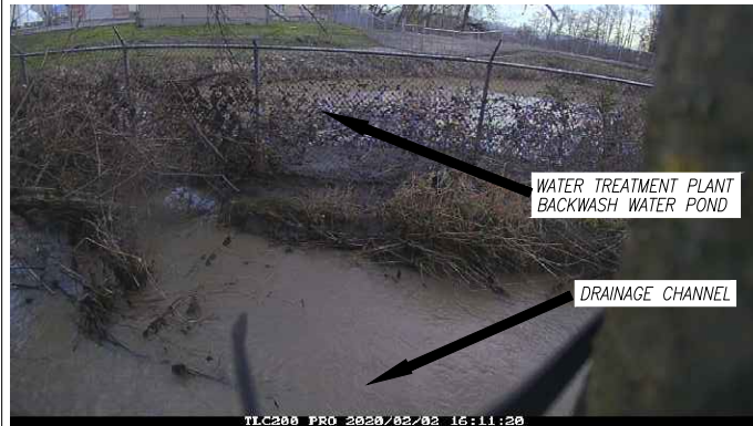
BANK EROSION AFTER FLOOD - FEB 2020
